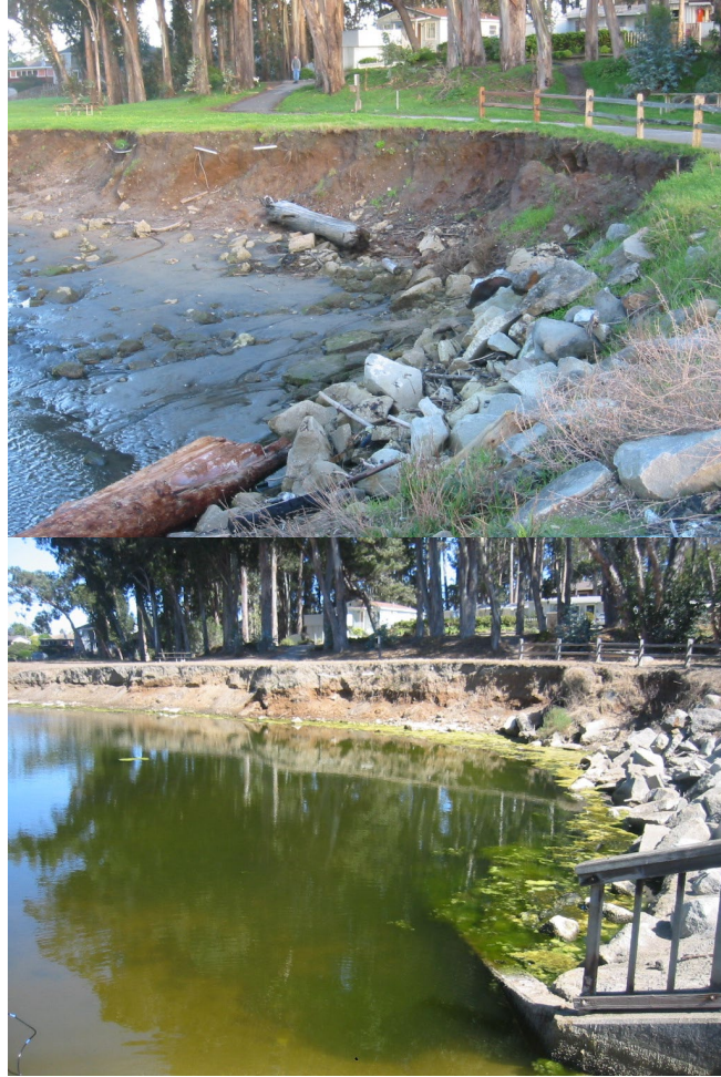
Figure 5.7. Eroding Bank on the Eastern Shore of Moran Lake (Photos taken on September 11, 2003 (lower) and February 2, 2004)
