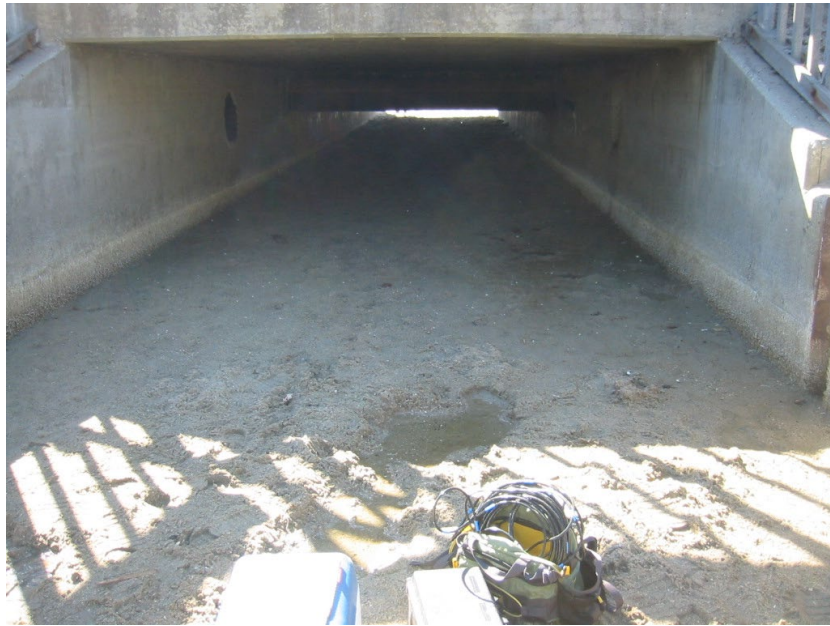
Figure 3.9. Moran Lake Box Culvert Closed with Sand– October 28, 2003
