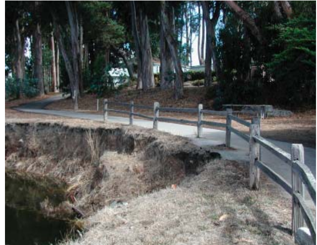
Existing Bicycle Path Compromised by Erosion (Figure 39)
