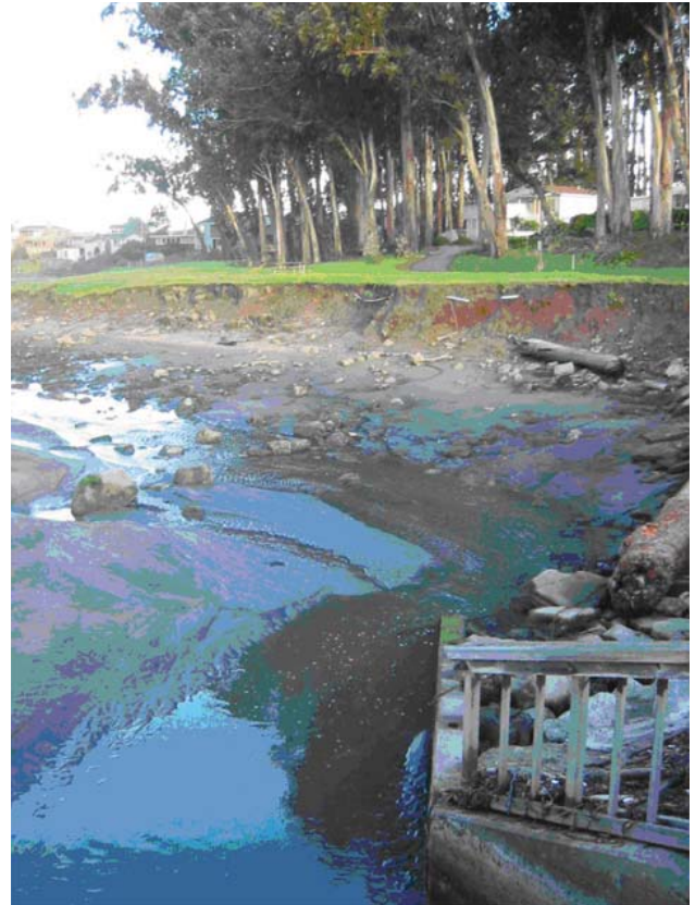
Eroding Bank on Eastern Shore of Moran Lake (Figure 21)
